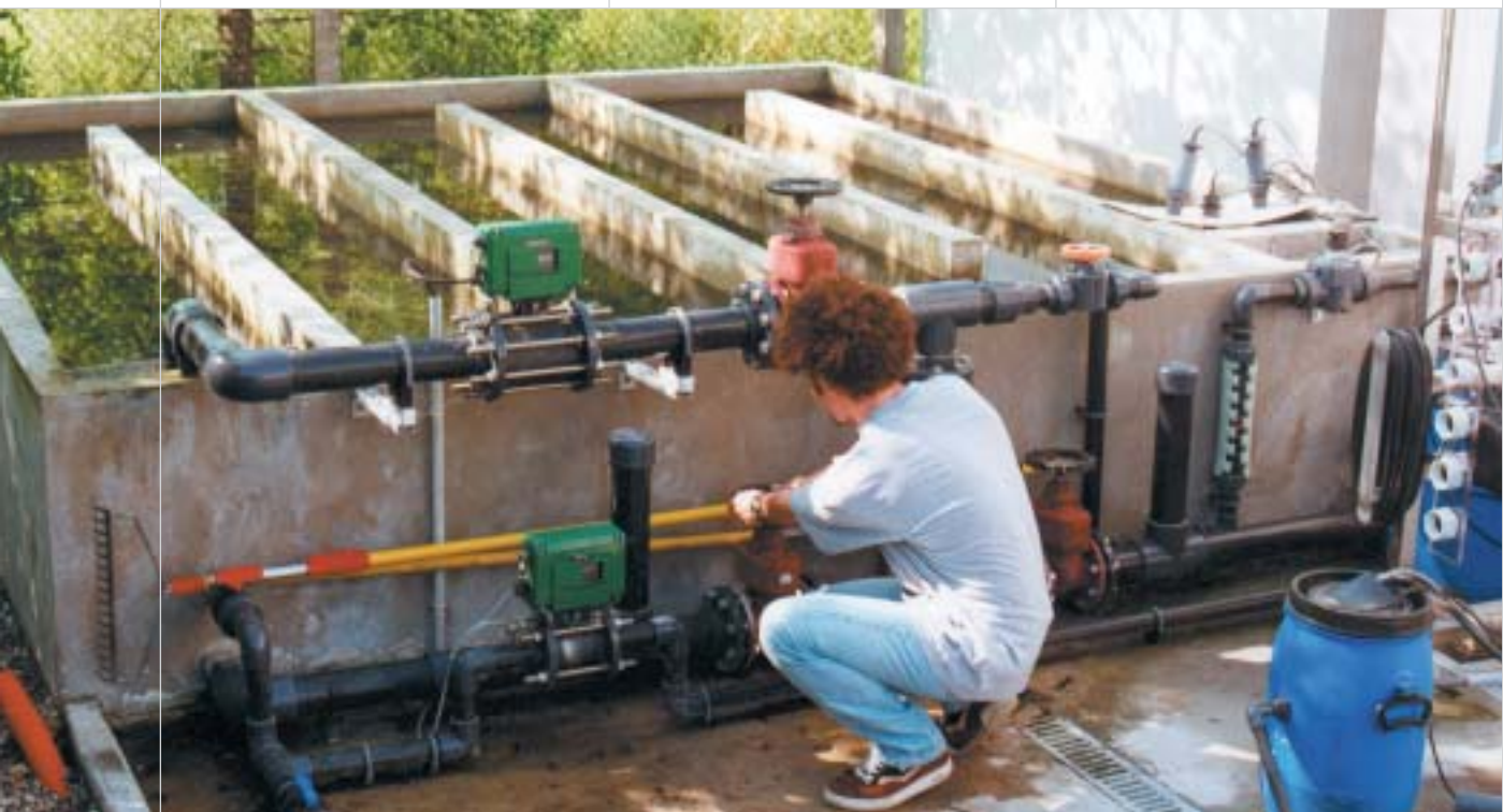
Organic treatment of waste water.
