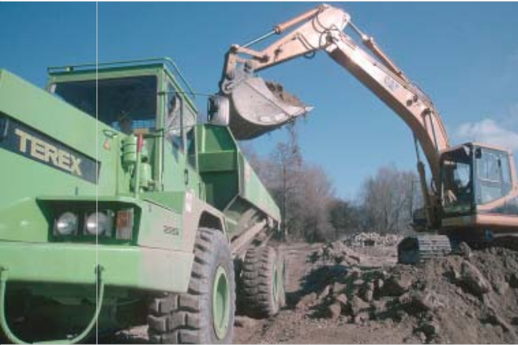
The works involved joining ox-bows of the river to the bed of the Danube.
